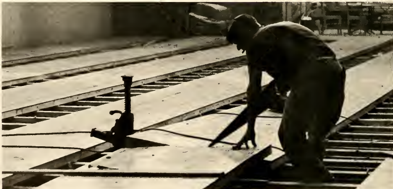
Craftsman removes bowling lanes in readying old union alleys for university book store.
